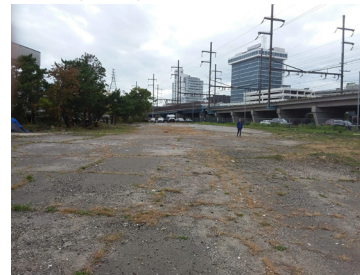
Degrading Asphalt Pavement
