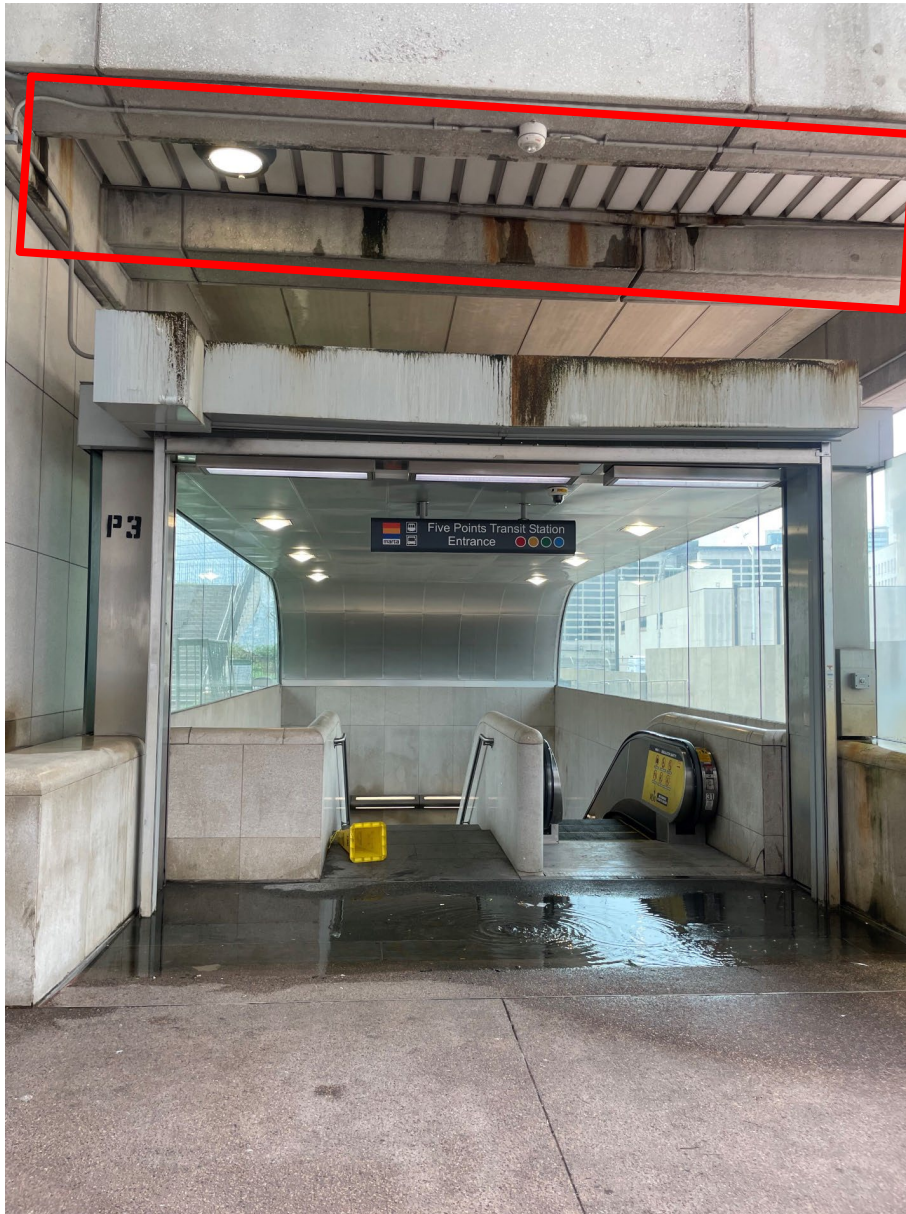
FIGURE 5. EXAMPLE OF THROUGH LEAKING DAYS AFTER A STORM EVENT THAT IMPEDES STATION MOBILITY
