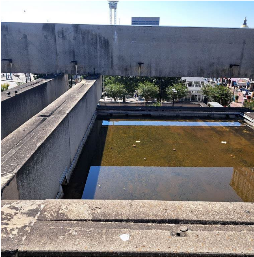
FIGURE 6. WATER RETENTION ON FLAT ROOF
