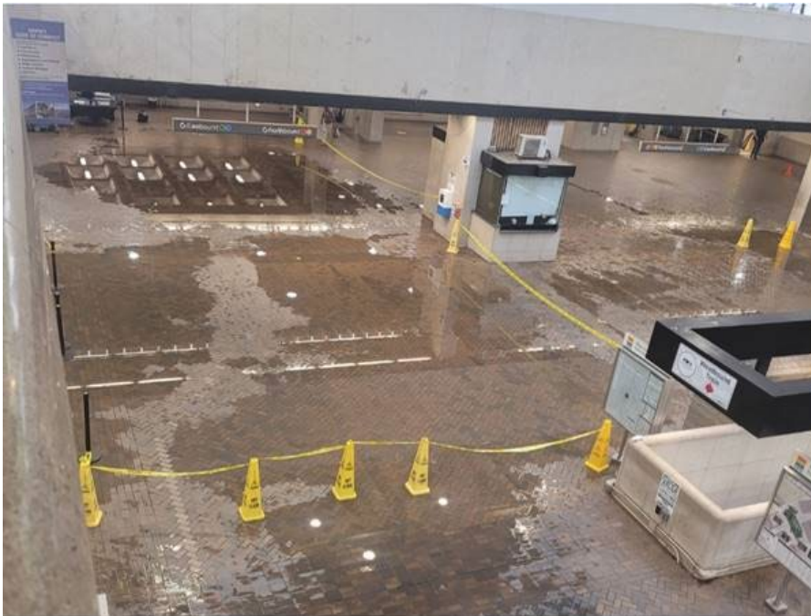
FIGURE 4. EXAMPLE OF WATER CONDITIONS ON THE CONCOURSE LEVEL AFTER A STORM EVENT
