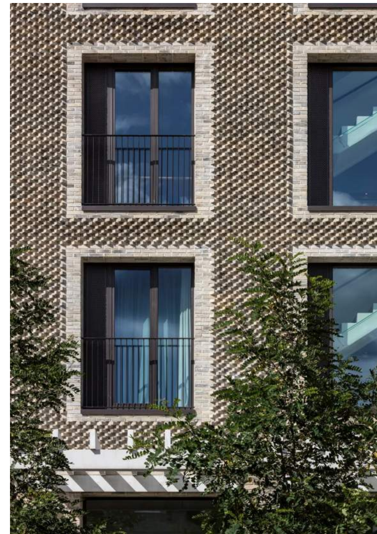
UNACCEPTABLE EXAMPLE CARLSBERG APARTMENTS CARLSBERG
